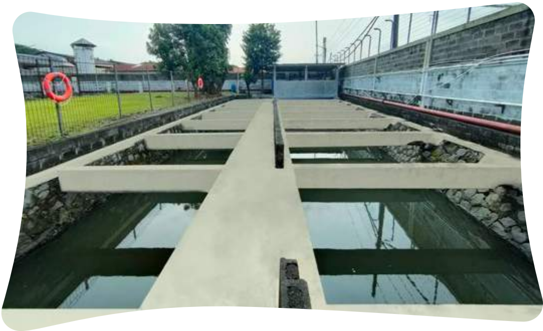
Rainwater Tank di Gudang Surabaya
